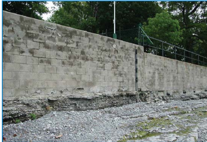
Figure C-3: Example of existing shore protection at risk of undercutting during low water periods
